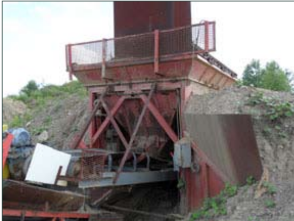
Hopper & Feed Conveyor to Deister
