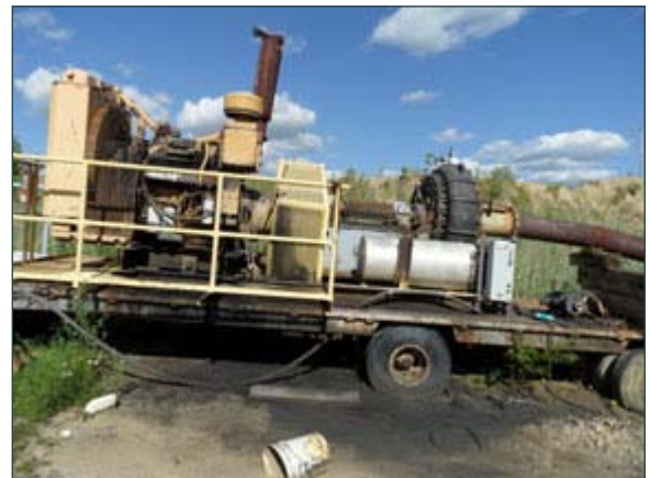
Thomas Booster Pump p/b Cat 3408
