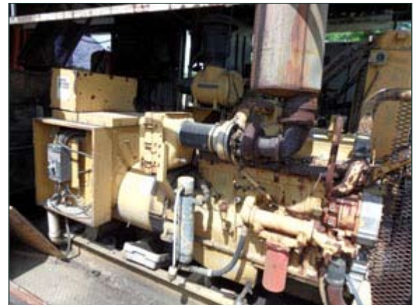
Cat Generator (on dredge)
