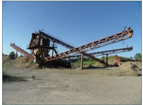
Deister Screening Plant
