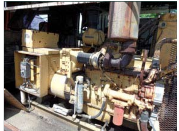
Cat Generator (on dredge)
