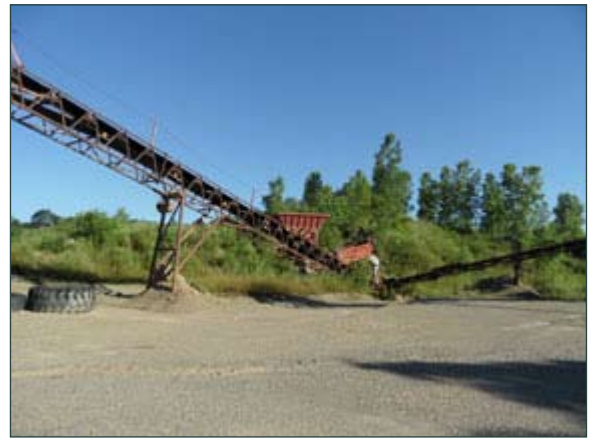
Coarse Material Wash Plant
