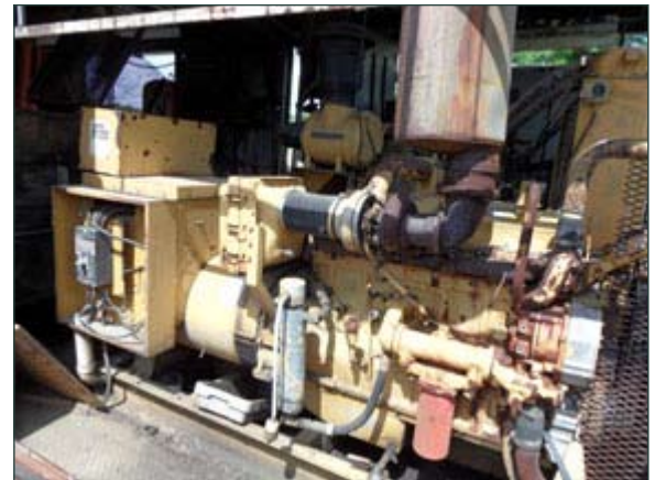
Cat Generator (on dredge)
