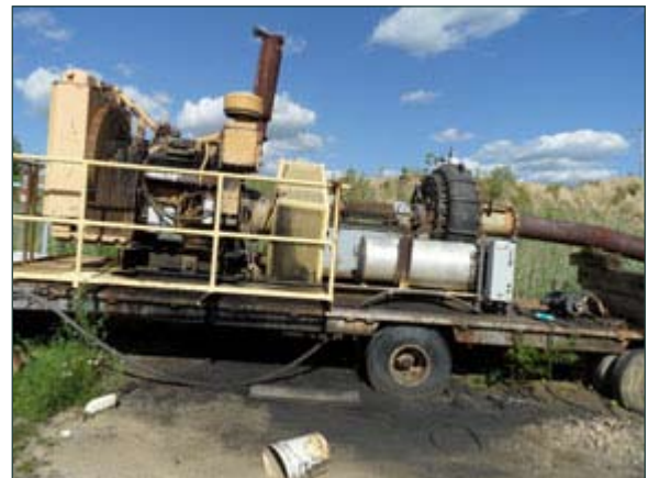
Thomas Booster Pump p/b Cat 3408
