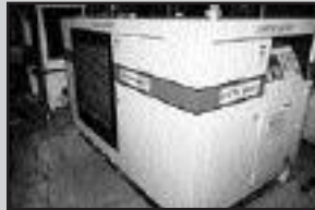
Gardner Denver 75 hp Compressor
